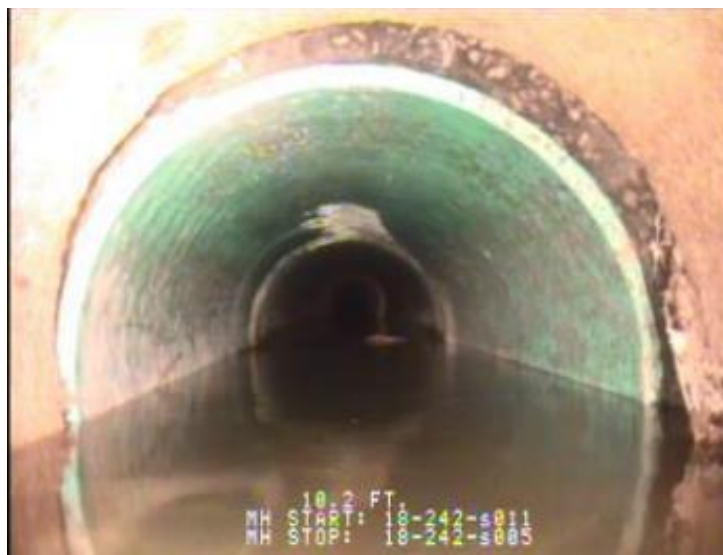
Evidence of Broken Pipe, and back-up
